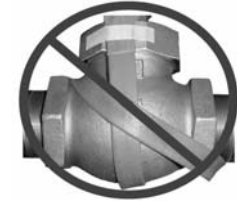
C.) Incorrect Installation: Heating tape overlapped on itself
